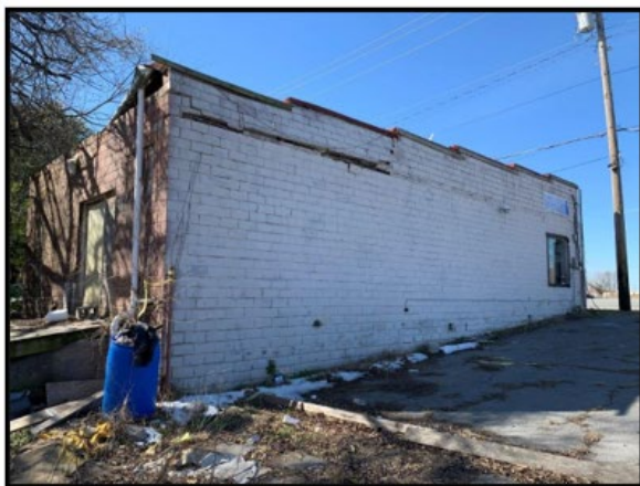
Photograph 10: View northwest of concrete block building on west side of subject property.
